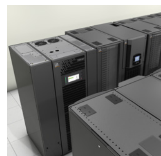
Liebert eXM adjacent to the wall
